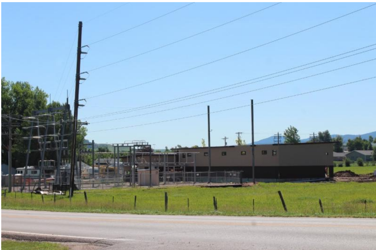
The new Black Hills Energy Operations Center at 455 Hillview Road continues to take shape with new siding and masonry completed in the last couple weeks.
