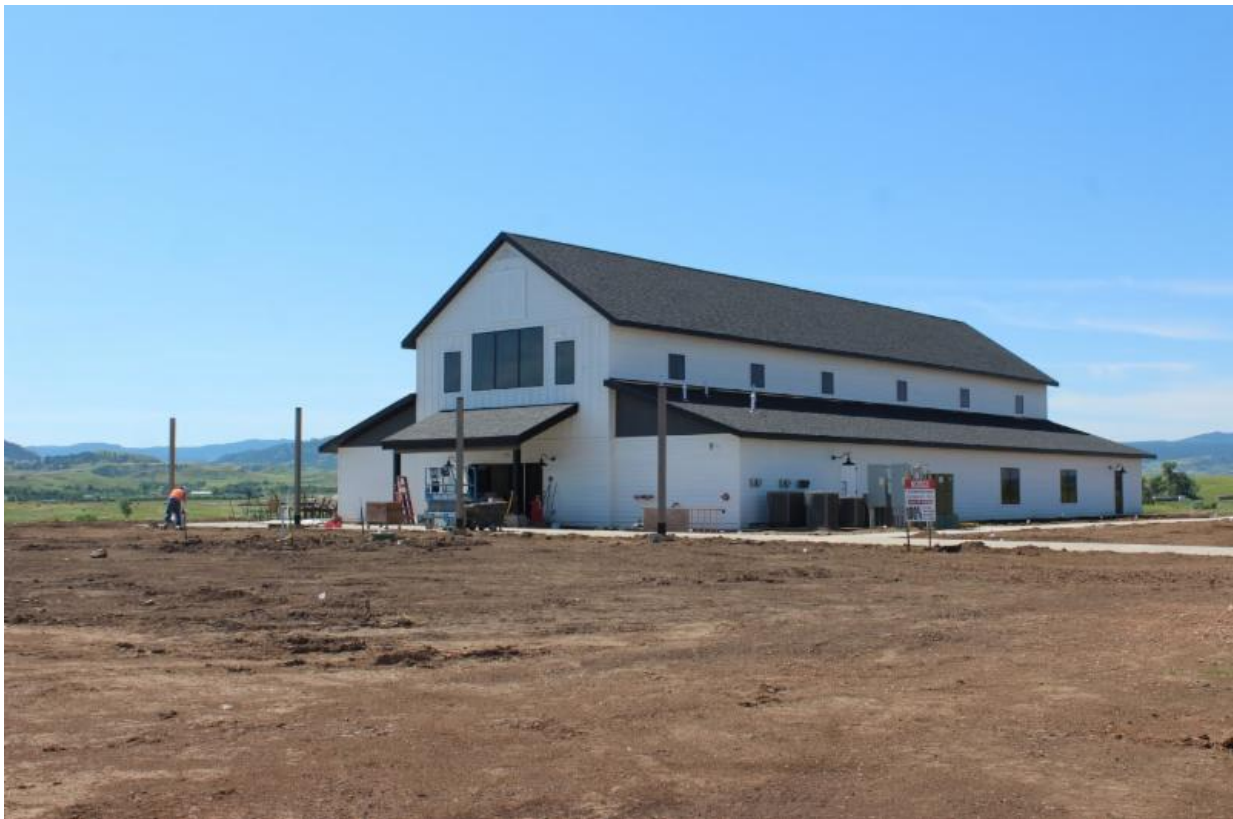
The Barn at Aspen Acres is set to be completed this week! Join us at their open house on September 7th from 4-8 PM.
