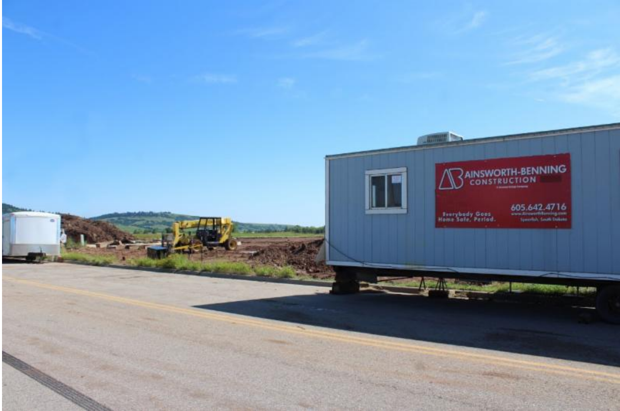
ONEOK, Inc. continues site work at their new location in the Spearfish Business Park. What a wonderful addition to our Spearfish community.
