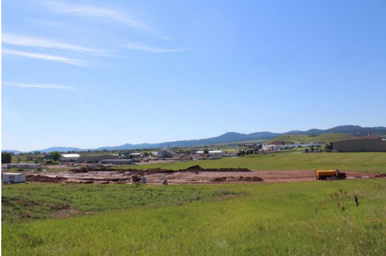
Infrastructure and dirt work continues at Access Point Development located in the Spearfish Business Park. This development has lots for sale!
