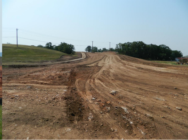
Infrastructure is being put in place for the new Miller Ranch Housing Development near Colorado Blvd!
