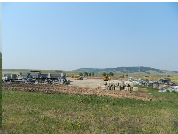
A new industrial facility will be constructed at the former Waupaca property in the Spearfish Business and Industrial Park!
