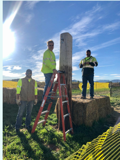
Butte Electric's Spearfish line crew volunteering at the Spearfish Corn Maze & Pumpkin Patch. They are installing the zip line to ensure a safe, fun ride for everyone!
